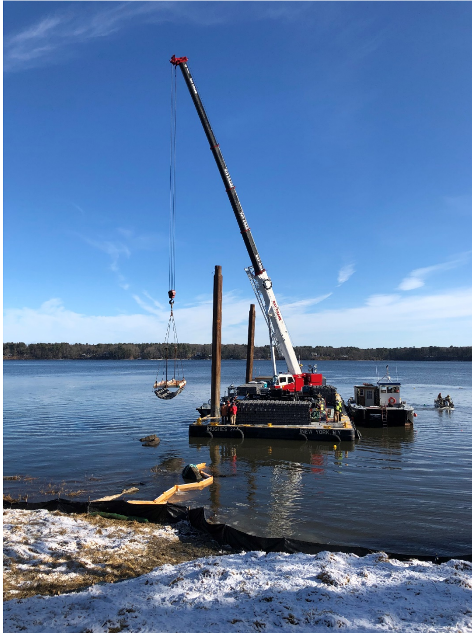
View from Getchell Property (Durham, NH) at the start of concrete mattress installation on the western tidal flat (12-11-19).
